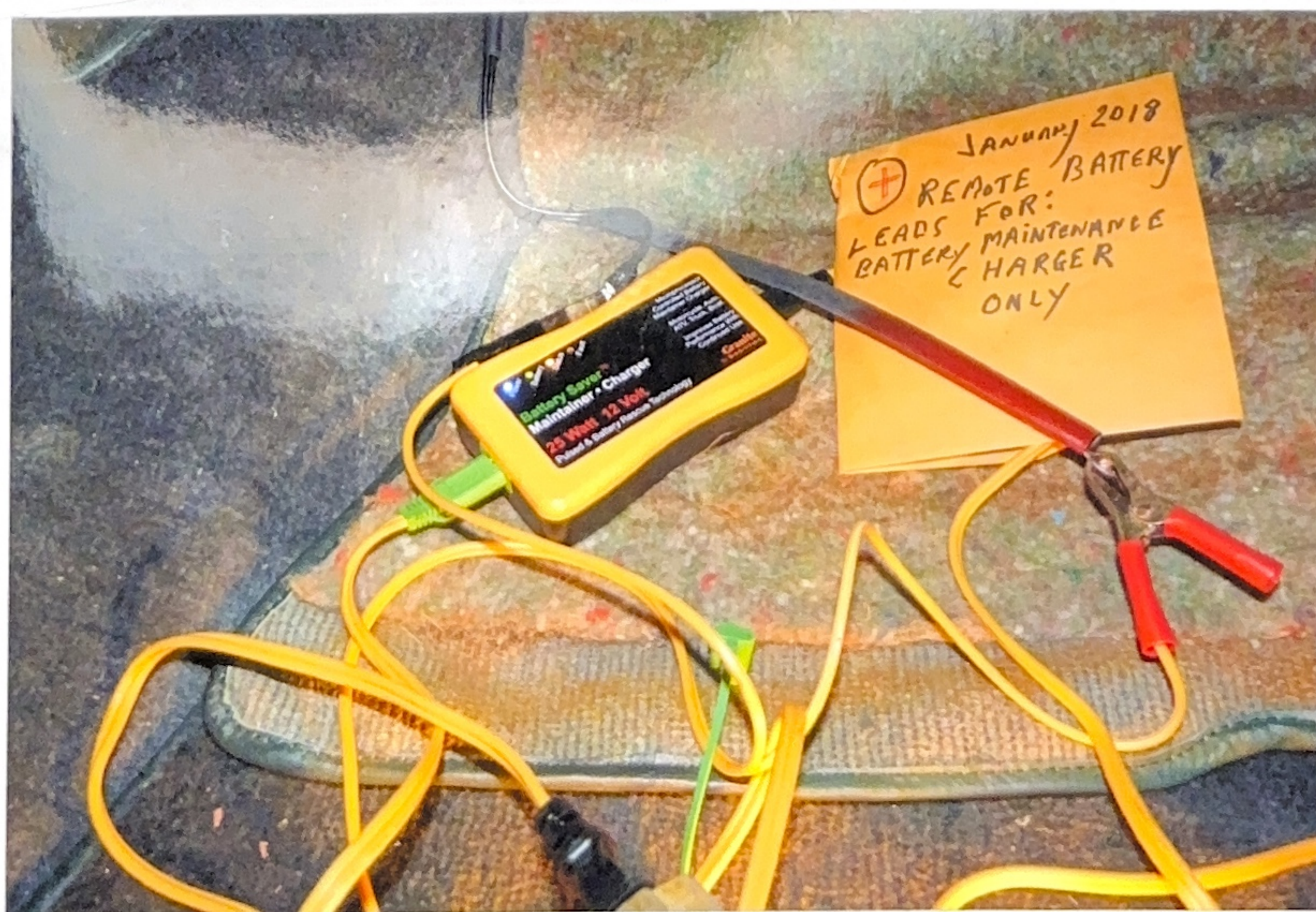
BATTERY GROUND SWITCH
