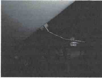
Poor repair on tank strap.
